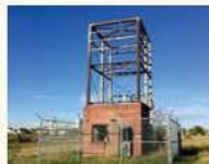
W3 Transformer station
