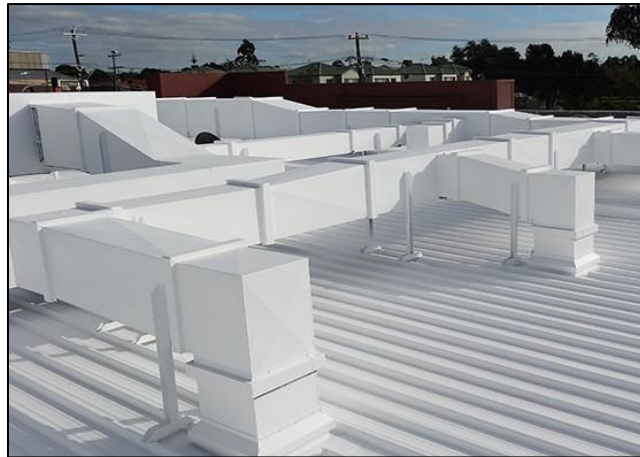
Camouflaging of rooftop equipment by painting the venting with a colour that is harmonious with the roof.
