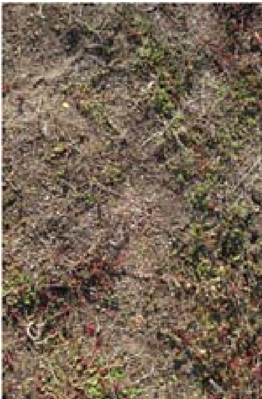
A8.4 Green Roof Service A8.4 Open growing medium exposed after weeding. A8.5 Wind erosion on local green roof
