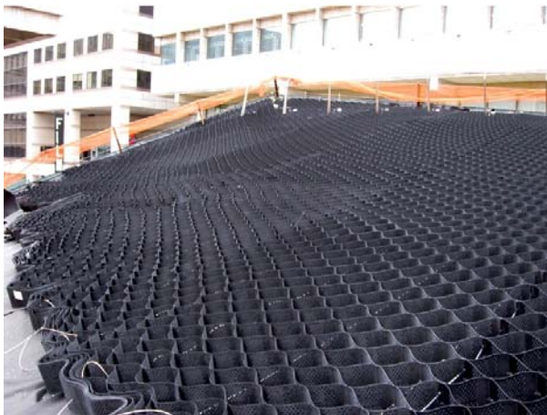
Figure 16.1: shows the application of a geogrid underlayment on the sloped green roof at Lincoln Centre in New York City.
