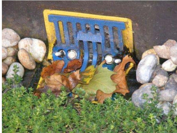
A8.9 www.maintenanceforgreenroofs.com A8.9 Blocked drain on a green roof
