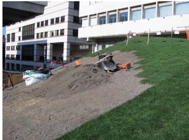
Figure 16.2: illustrates the subsequent steps in the Lincoln Centre green roof of applying the growing medium into the geogrid and laying sod on top.
